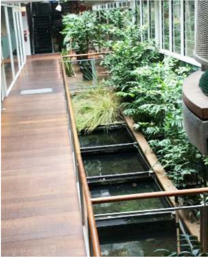
Water filtration system at 60L Leicester Street
